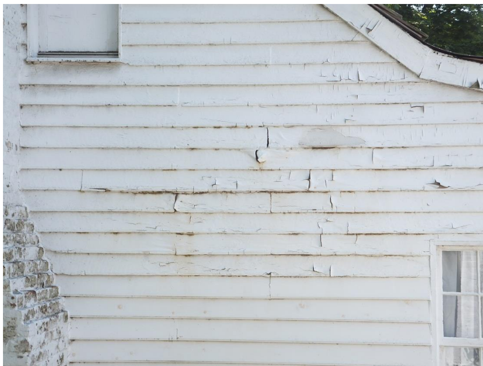
Before restoration, showing peeling paint on siding, railings, doors, and chimney.
